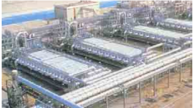
Figure B-4: Aerial view of a large Multi Effect Distillation Plant
