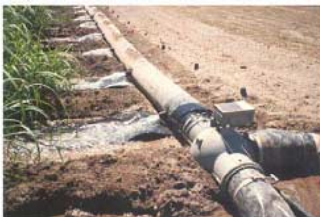
Figure 2 Surge valve installed at site 5
